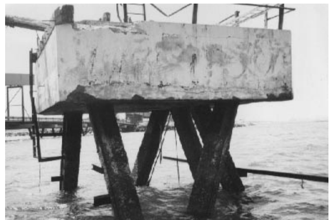
Figure 6: Damaged concrete structure
